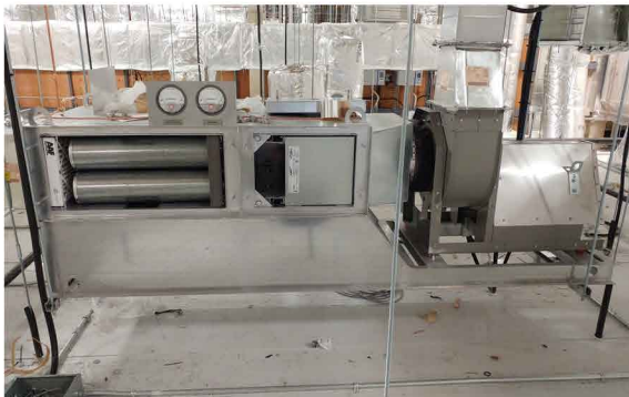
HEGA-HEPA Filter Fan System (Carbon Canisters & HEPA Filters)
