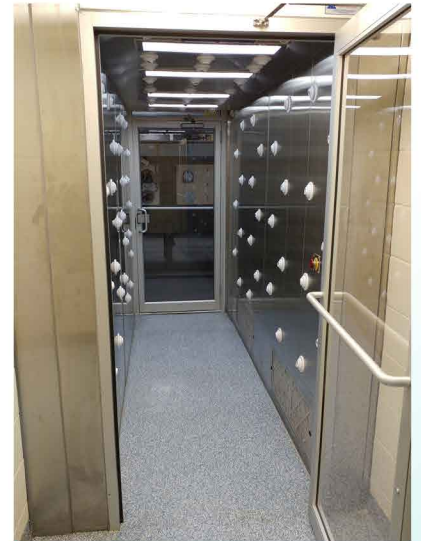
Air Shower Tunnel
